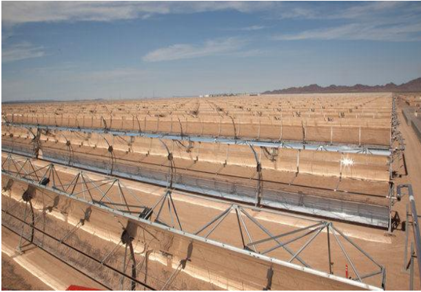
The trough-shaped mirrors of the Solana project in Arizona.
